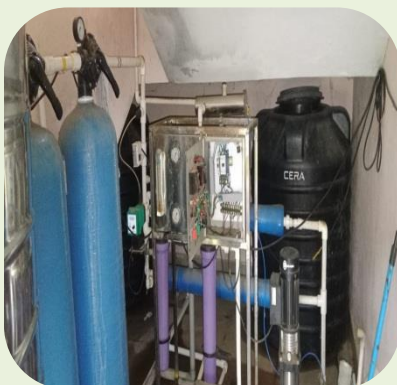
R.O. WATER PLANT
